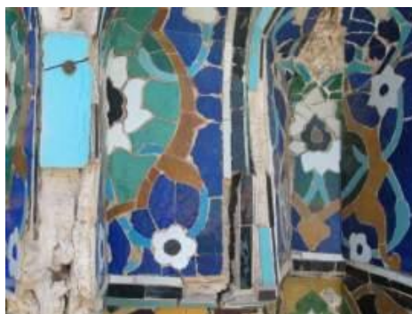
Figure 19 - Inappropriate Mortar (Writer)
